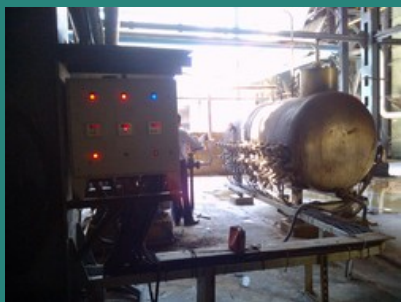
Super Heater Water Wash System
