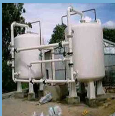
Groundwater Treatment System
