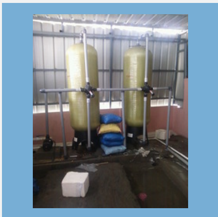
Reverse Osmosis Plant
