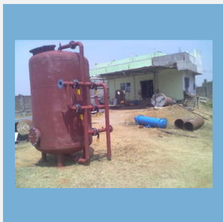
Pressure Sand Filters
