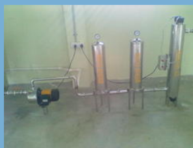
Water Filtration System
